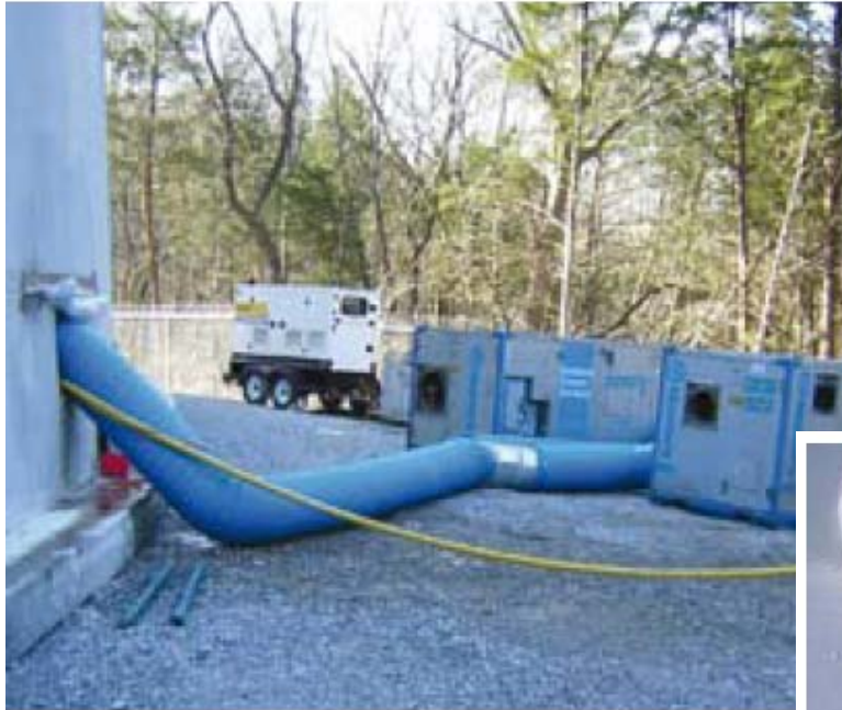
Flexible ducting is utilised to efficiently distribute the dried air within the tank.
