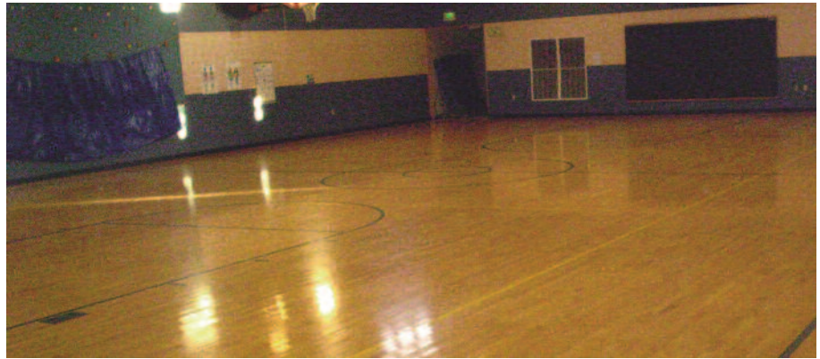
Directly Above: Two Munters DryCool units were installed on the roof of the school to correct the moisture problems and successfully salvage the gym floor. Top: The school is built into the side of a hill, exposing the exterior walls to moisture trapped in the soil.
