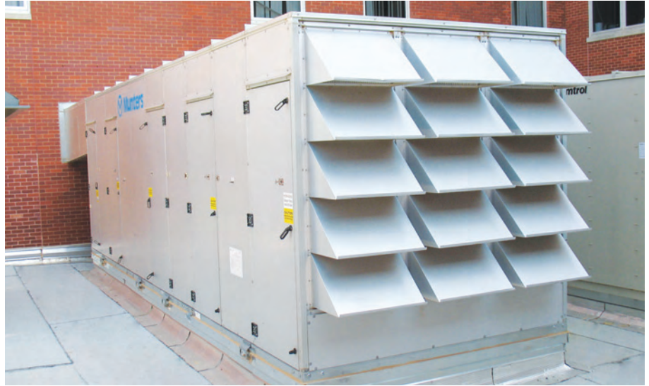
Above: The desiccant dehumidification system installed, will not only provide cost-efficient temperature and humidity control, but also a more comfortable environment for doctors, staff, and patients.
